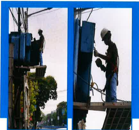
Ensuring the Power Supply Uninterrupted even During the LOCKDOWN #ContinuingEssentialServicesinCorona
